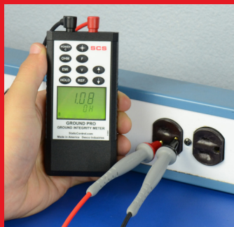
Measuring Ohm Impedance between Neutral and Ground
